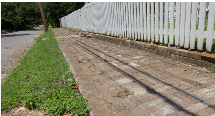
Brick used in sidewalk (716 Belvin St)
