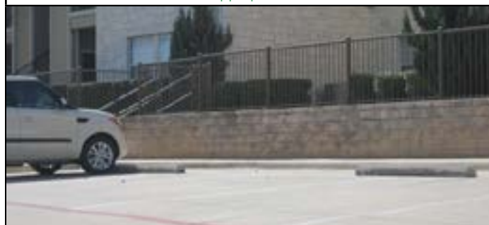
Curb stops for parking spaces directly adjacent to sidewalks: appropriate
