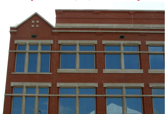
Horizontal expression: cornice, window sills and moldings. Cornice; Window-Design includes sills and insets
