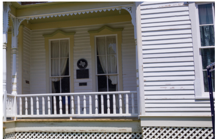
Horizontal wood siding is the most common exterior wall surface (716 W Hopkins St)
