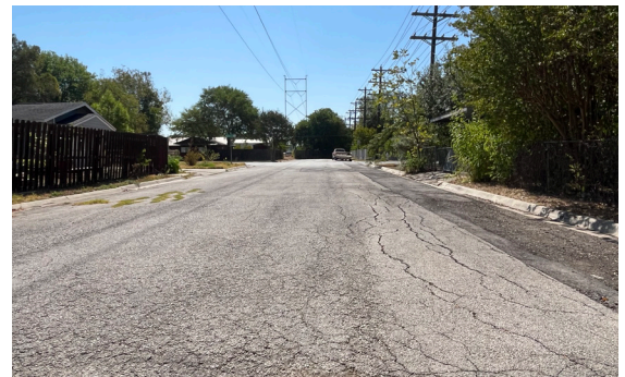
Cracked asphalt along Highline Drive.
