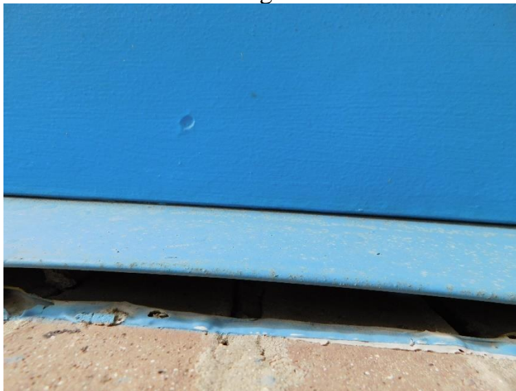
Exterior wall flashing allows water to enter structure
