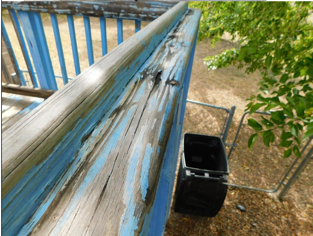
Rear porch railing damage
