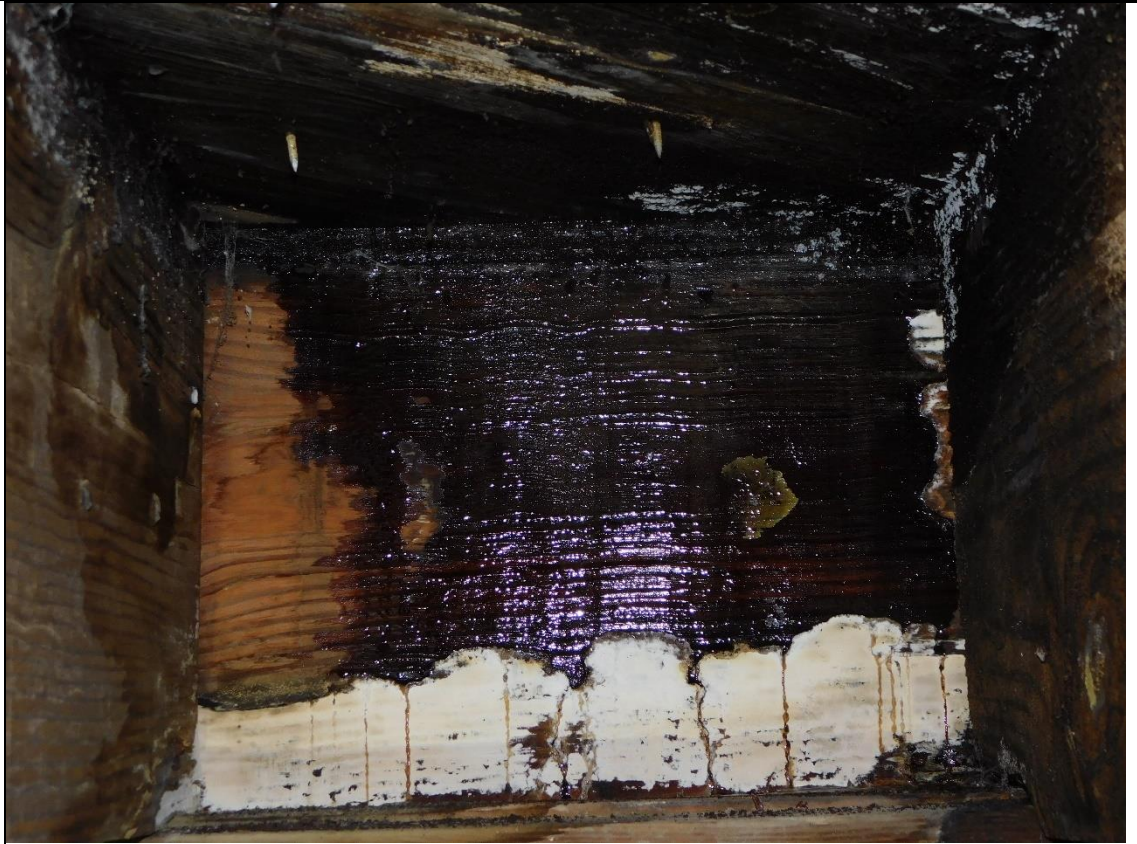
Black mold present with active water leak/subfloor damage
