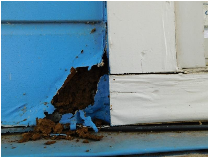
Exterior wall water damage to Masonite siding
