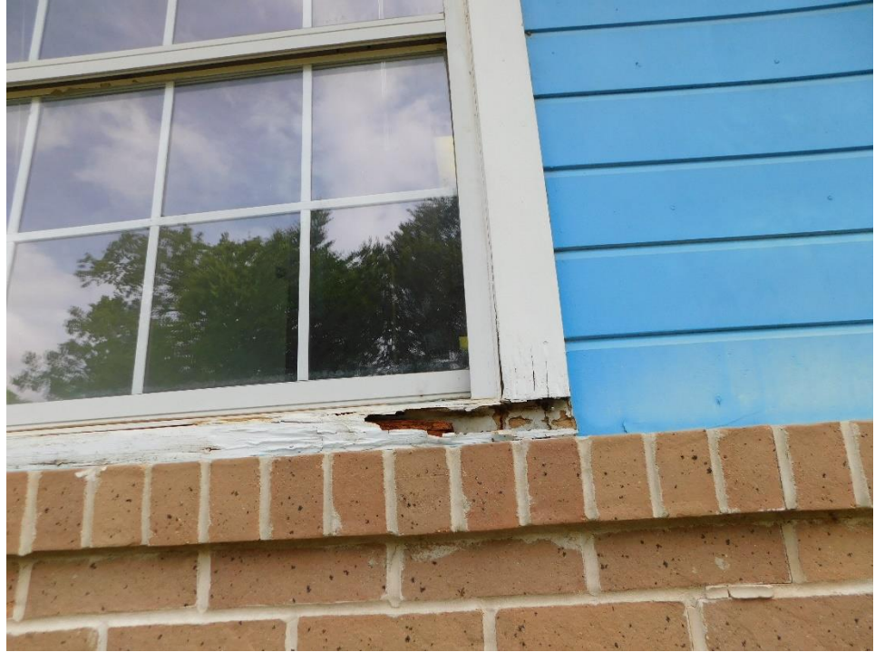
Exterior window trim damage
