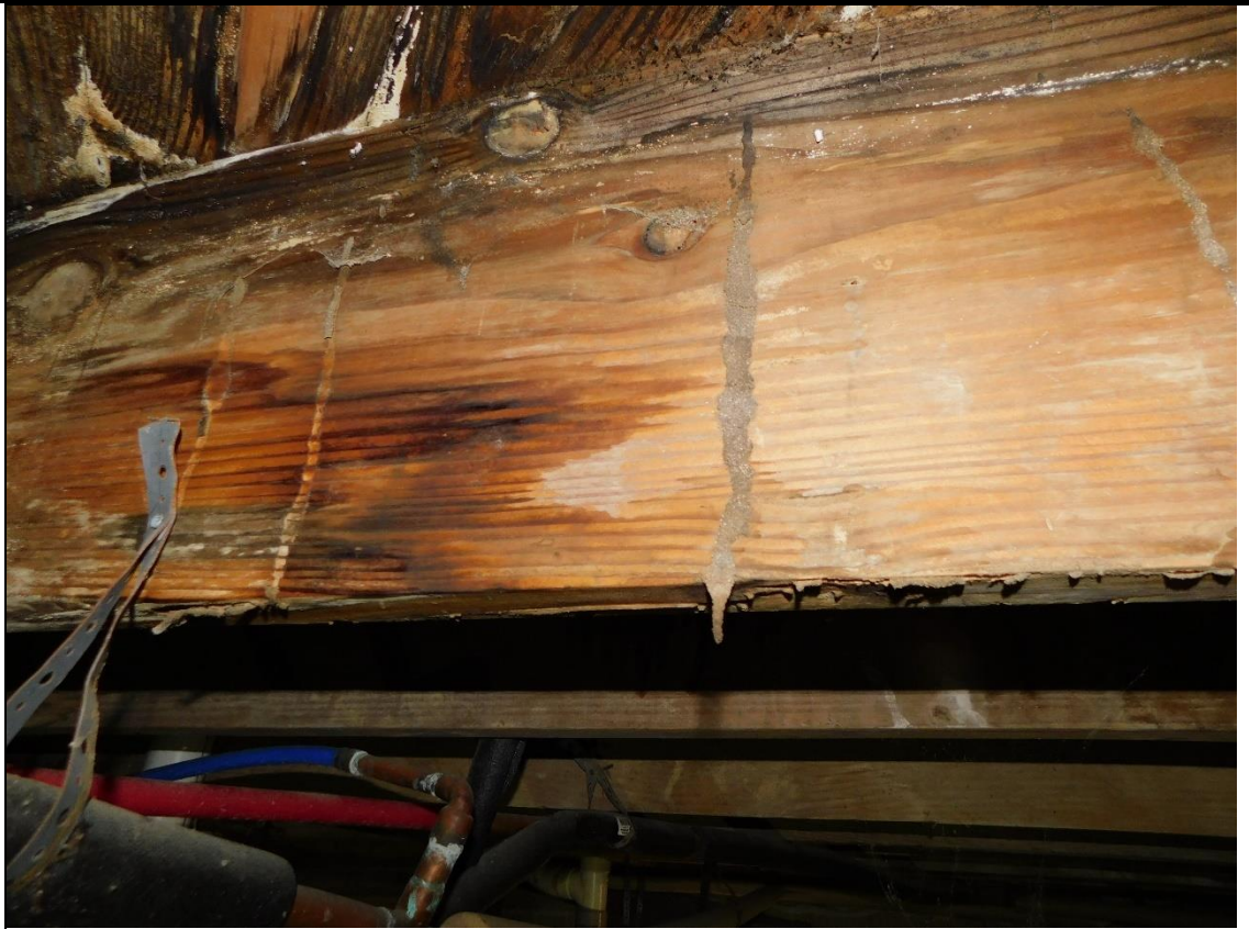
Termite shelter tubes on floor joist
