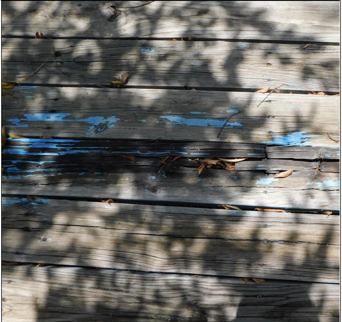
More decking damage
