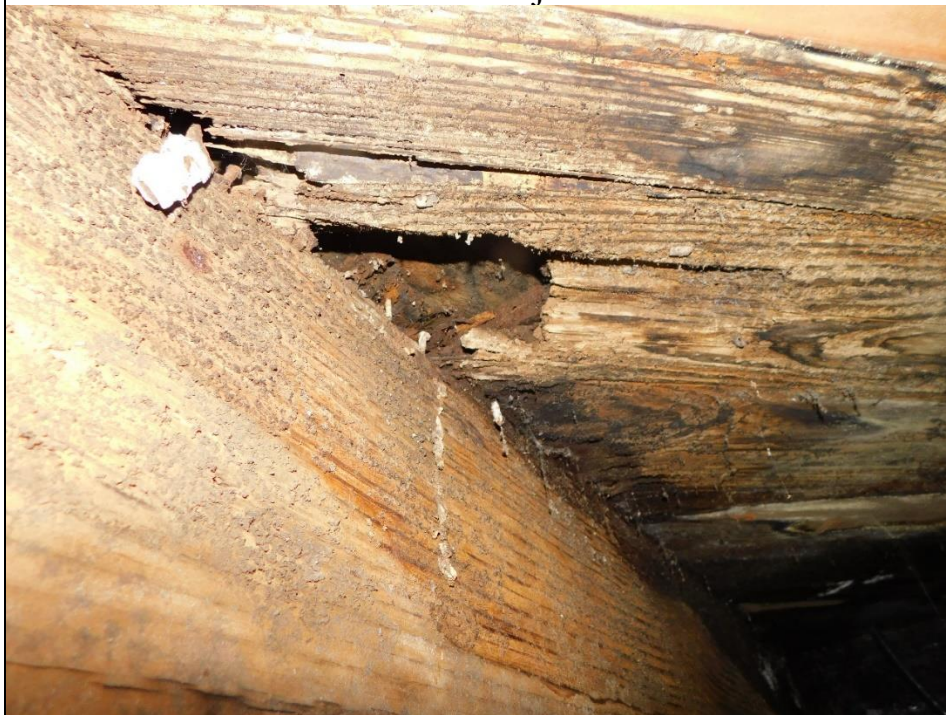
damage to floor joist and subfloor
