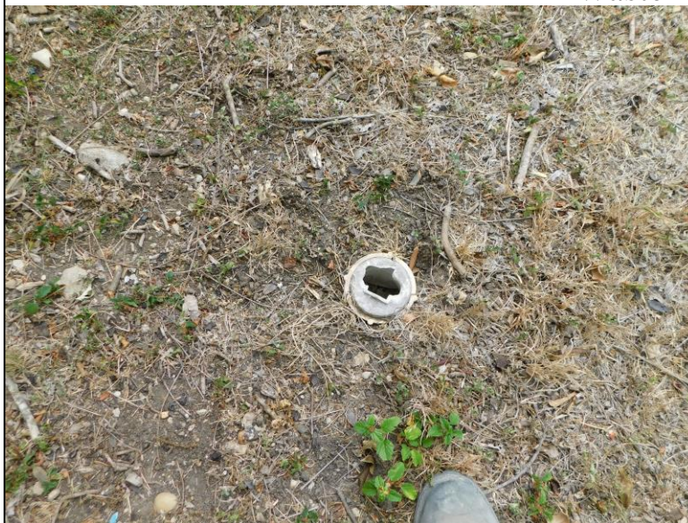
Damaged clean out
