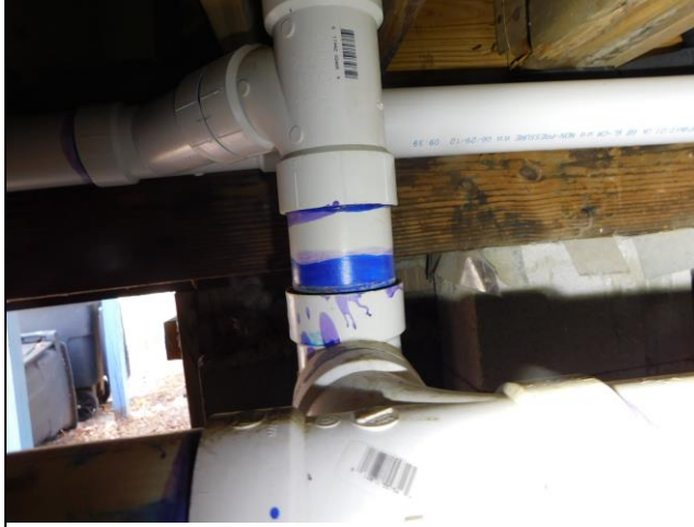
Waste Pvc pipe
