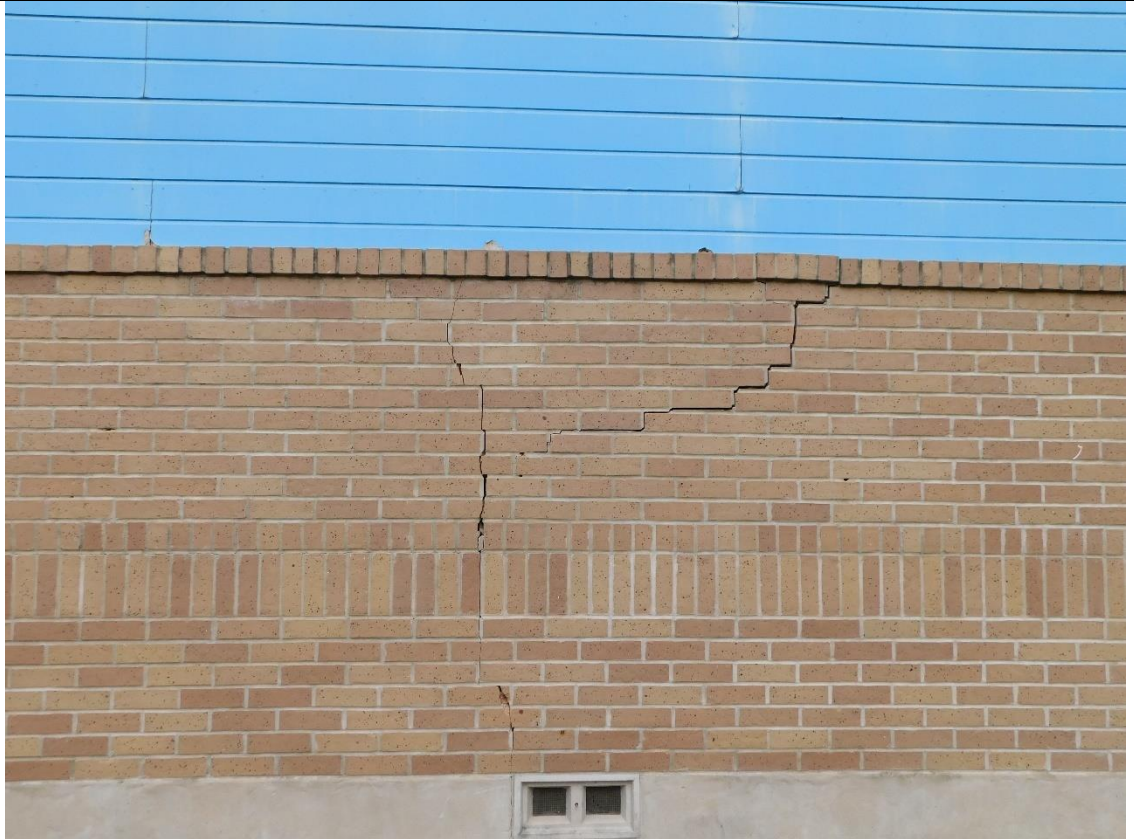
More wall stress cracking
