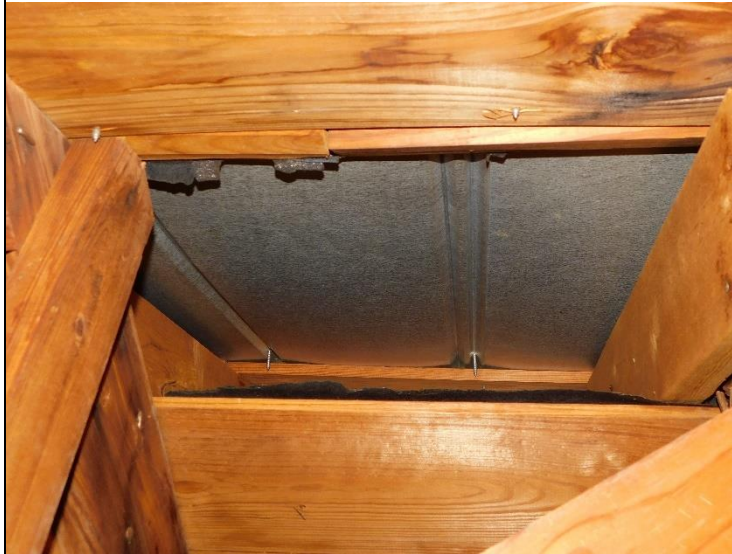
Various roofing fasteners do no secure to joists
